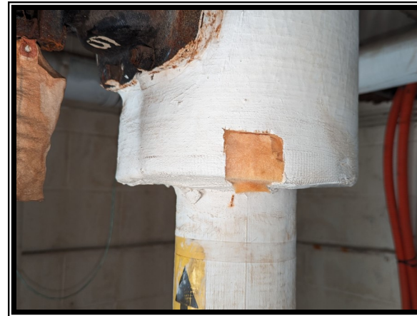
Photo #12 No Asbestos Detected in Boiler Pipe Wrap or Mastic Materials
