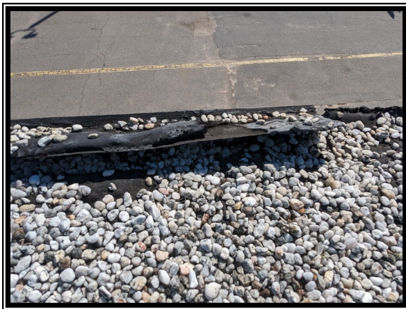
Photo #7 Asbestos Detected at 5% in Sealant Layers of Perimeter Flashing on Roof Section D
