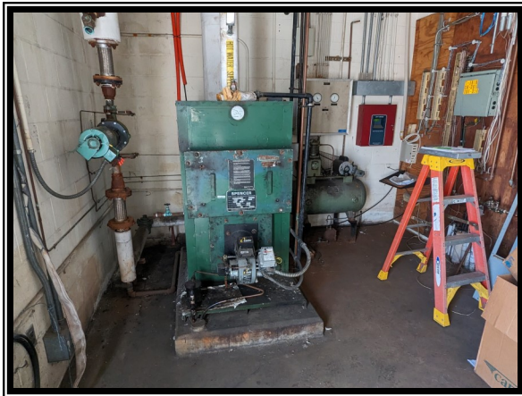
Photo #11 View Depicting Boiler Equipment in Boiler Room
